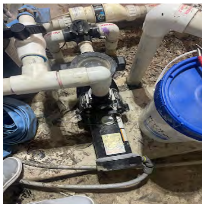
Bad Filter Pump Motor
